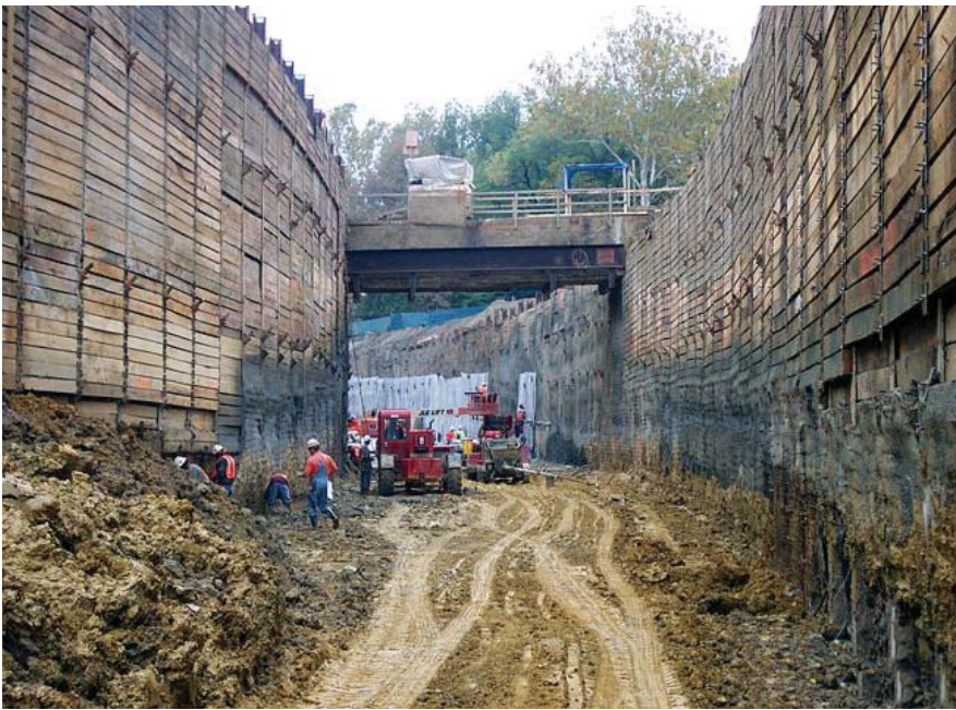
Originally a company dedicated to pile driving, Subsurface has made itself into a leader in foundation and earth retention work. Here, a retention system the company built for Metrolink.
