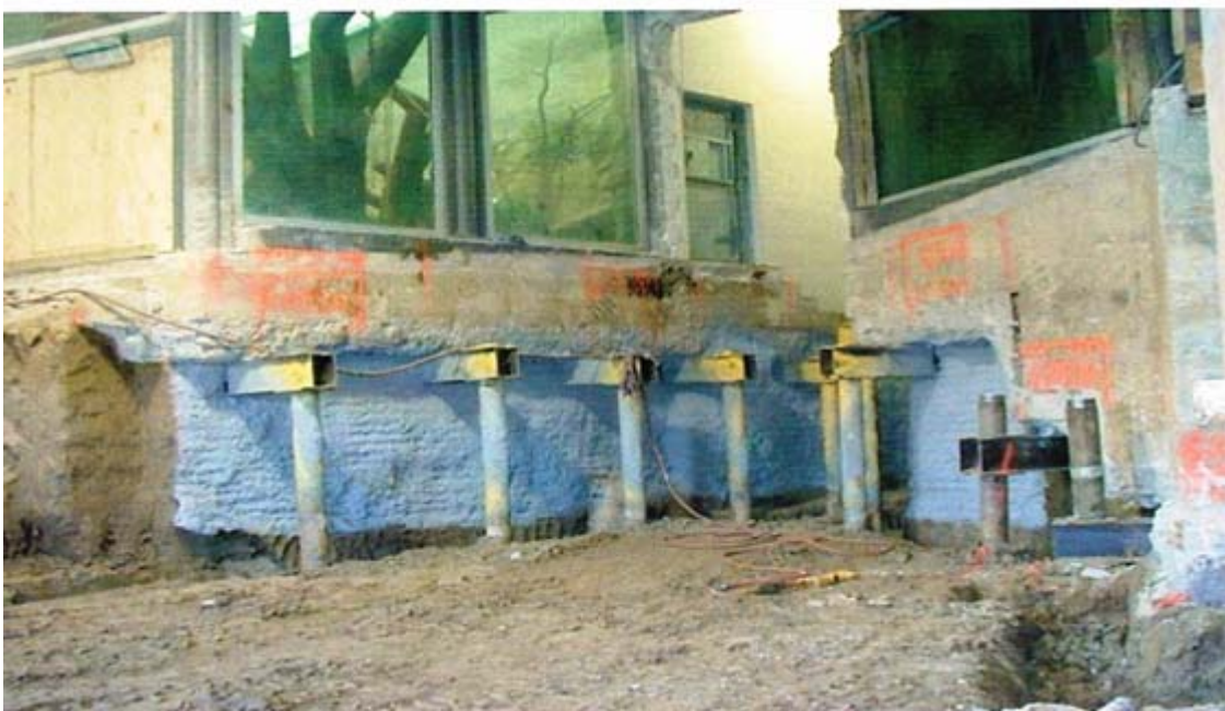
St. Louis Zoo Fragile Forest, St. Louis, MO – Micropile for Underpinning Existing Building
